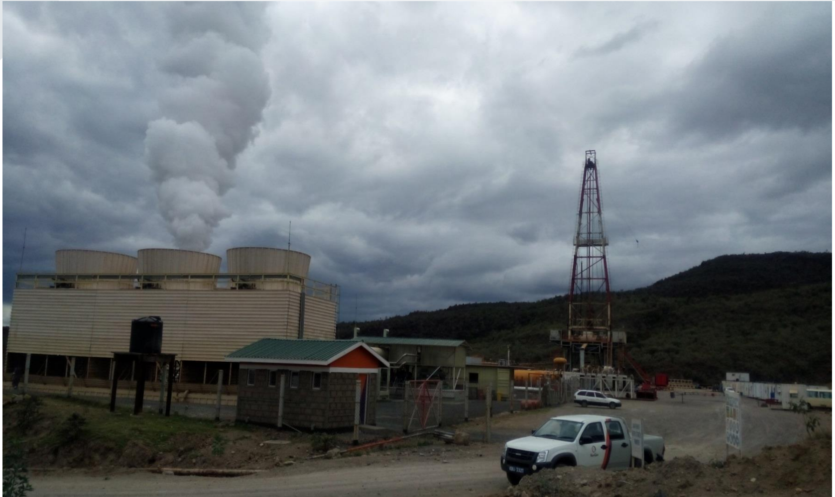
Fig. 2. Wellhead Plant OW-37 with rig KGN02 drilling on the same well pad.
