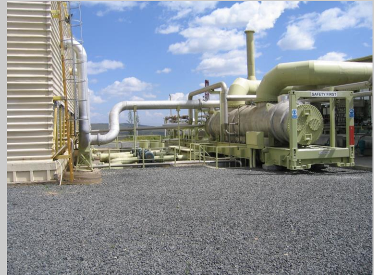
Wellhead unit at Olkaria during ArGeo 2012 tour
