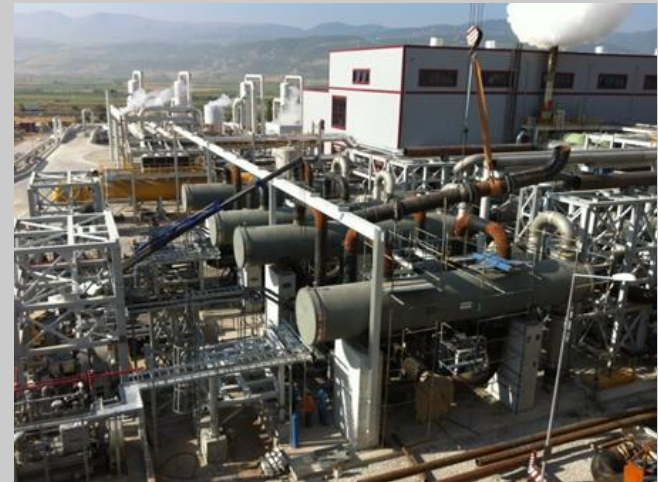
80 MW Kizildere-2, water-cooled combined cycle
