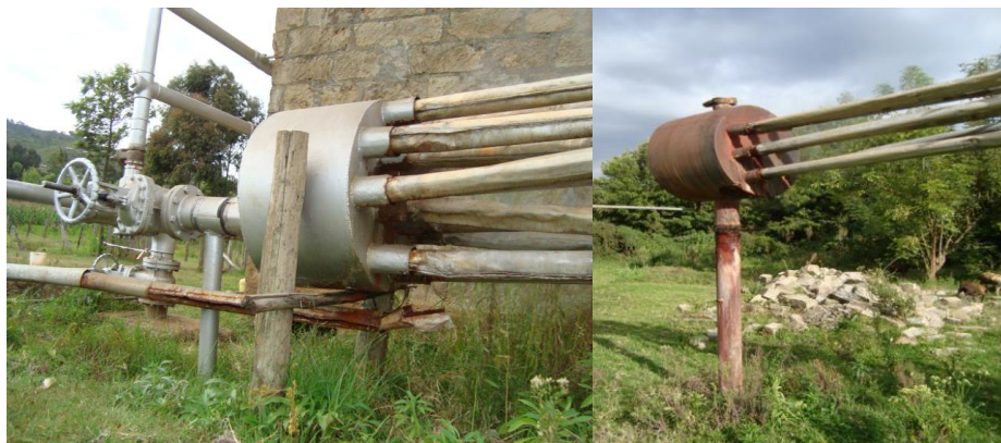
Figure 4: Two Shallow steam wells at Ex Peter-Eburru drilled in 1950s
