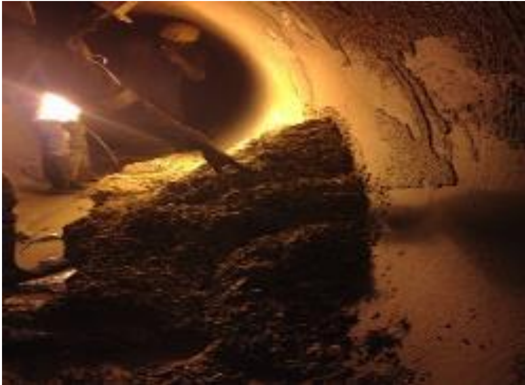
Figure 11: Deposit of foreign material in the cooling tower GRP pipe
