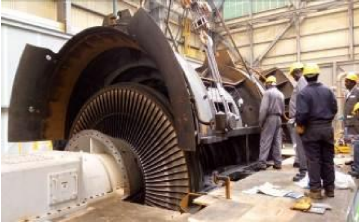
Figure 9: Steam turbine inspection
