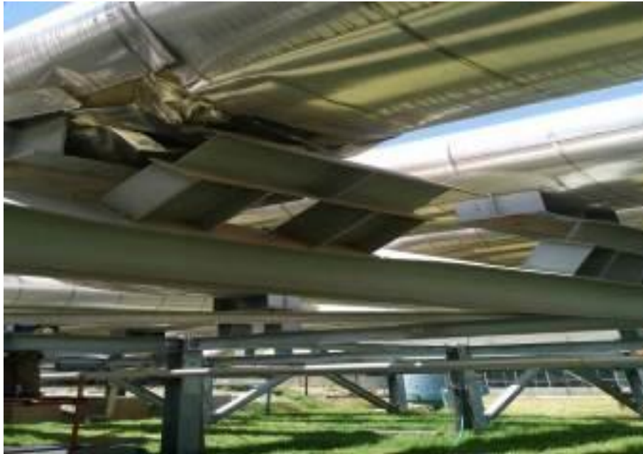
Figure 7: Deflected main steam line supports
