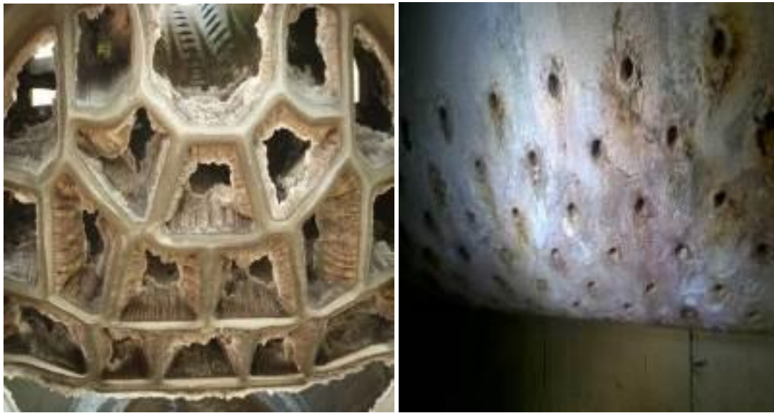
Figure 6: Clogged vent valve and diffuser
