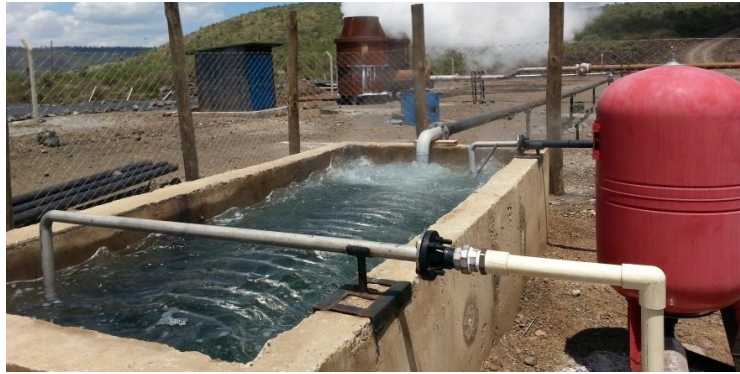
Figure 2: Water bath heat exchanger
