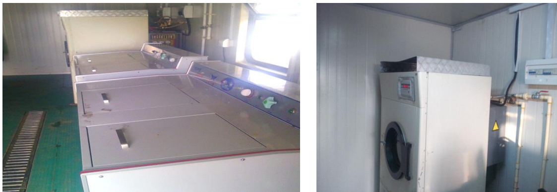
Figure 6: Geothermal Heated Laundromat.
